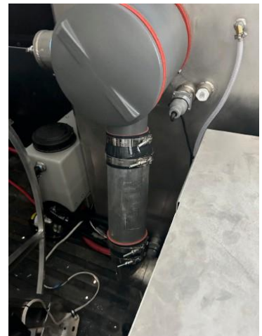
Aluminum tube to the blower inlet and waste tank inlet.
